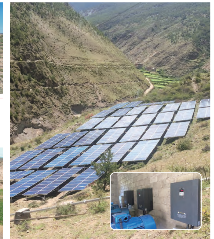
160kW Controllers: 4*PDS33-4T037 Location: Sichuan Province, China
