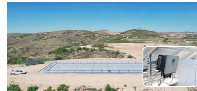
4.8kW Controller: 1*PDS51-4T2R2-E Location: Shanxi Province, China
