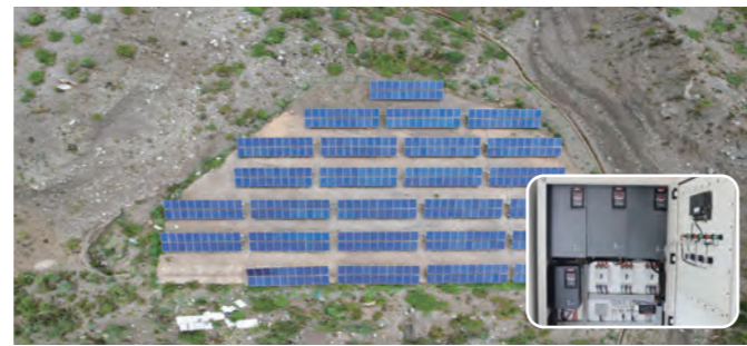
143kW Controllers: 3*PDS33-4T030 + 1*PDS33-4T015 Location: Sichuan Province, China
