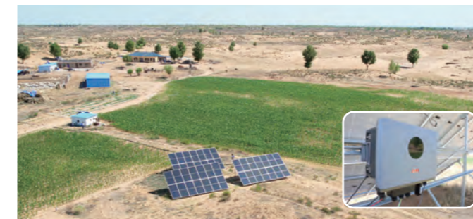
18.9kW Controllers: 3*PDS51-4T004-E Location: Inner Mongolia, China
