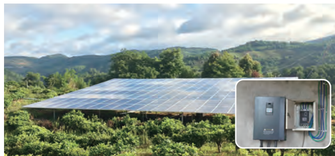
98kW Controllers: 2*PDS33-4T037 Location: Yunnan Province, China
